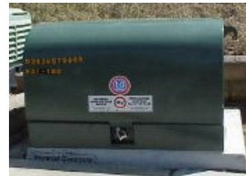
Pad-Mounted Single-Phase Transformer
